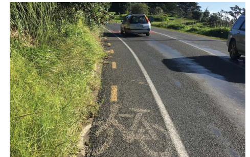
Oceanview Road - narrow cycleway with loose gravel
